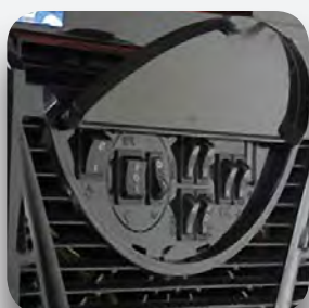
Panel de control.
