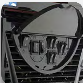
Panel de control.
