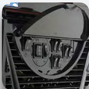
Panel de control.
